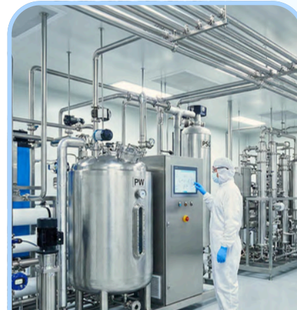
Water System & Utility Piping
