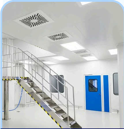
Cleanroom Wall & Ceiling Panels
